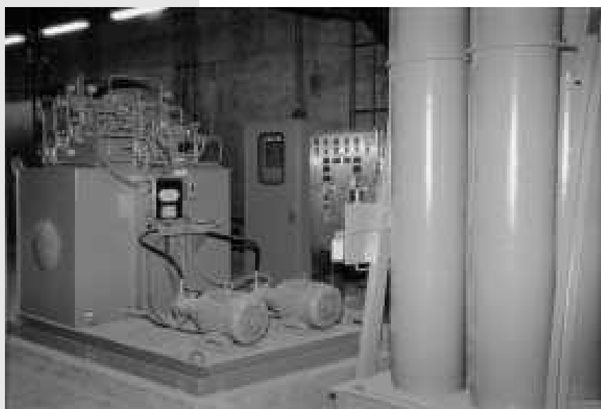
This Rodney Hunt hydraulic actuation system operates two 156 " x 192 " Rodney Hunt crest gates installed at the Deer Island facility in Boston Harbor.
