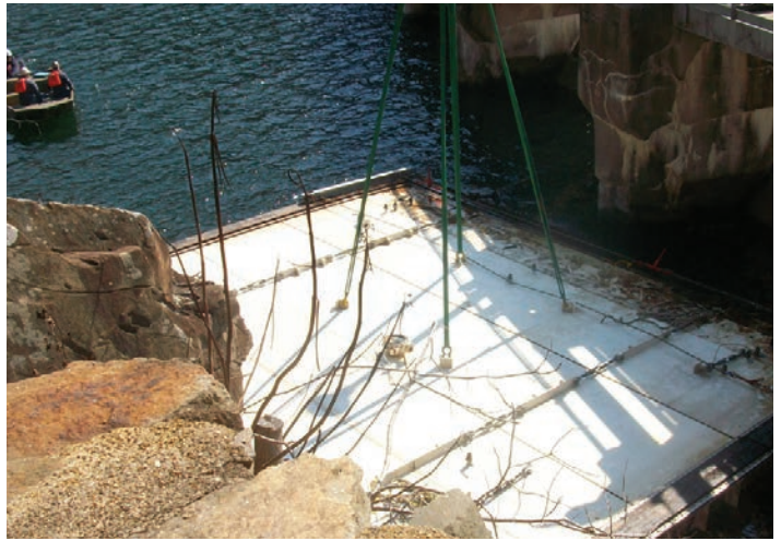
After some re-engineering to compensate for the degradation of concrete discovered after dewatering, the floating bulkhead is again lowered into the water upstream from the dam.
