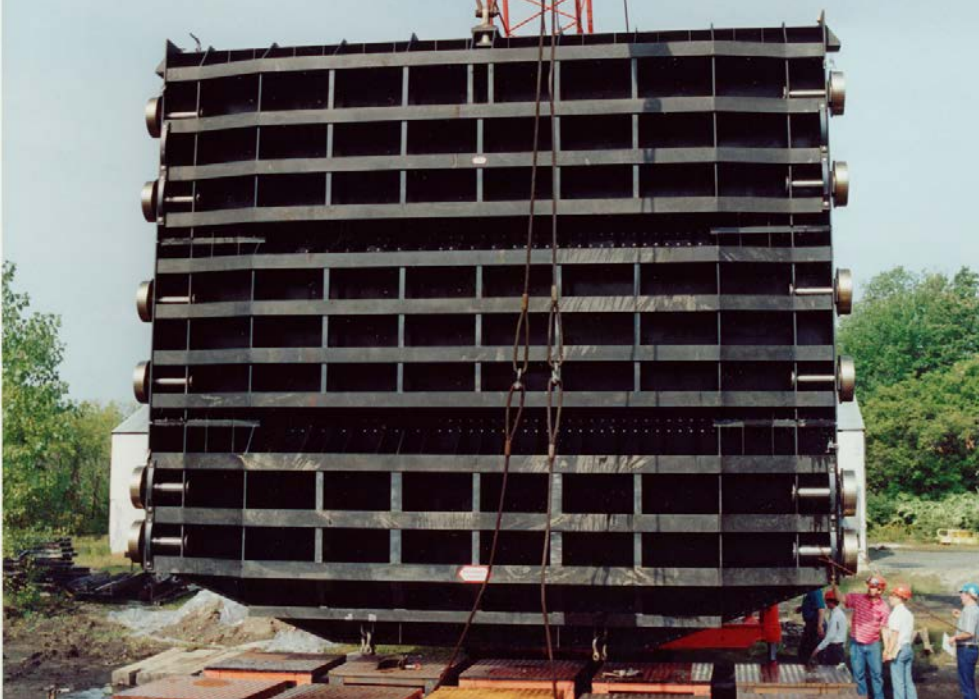
This 30' x 28.5' fabricated steel roller gate was installed at Idaho Power's Swan Falls Hydroelectric facility.
