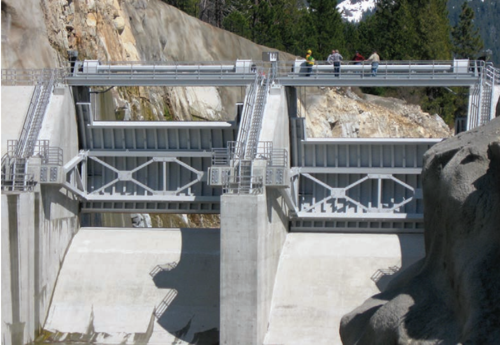
Two 36.5' x 18.85' Rodney Hunt Tainter Gates have been installed at the L.L. Anderson Dam.
